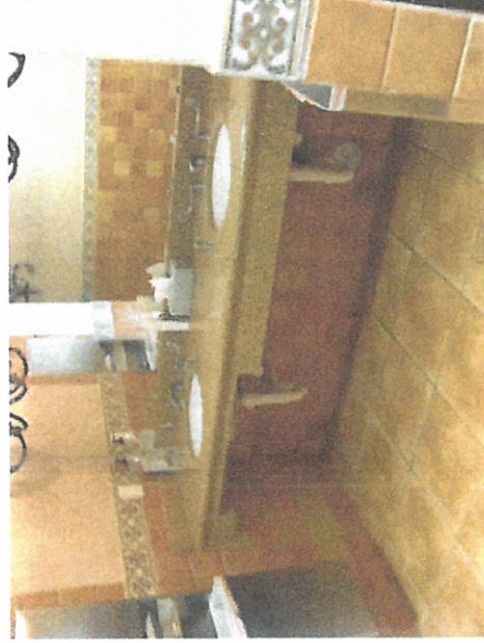
Vanity and sink
