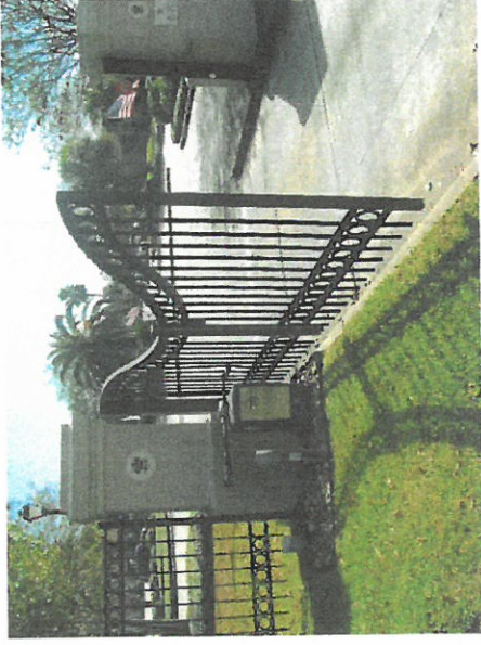
Gate and operator
