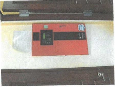
Life safety system control panel
