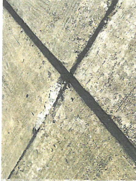
Concrete spall at joint
