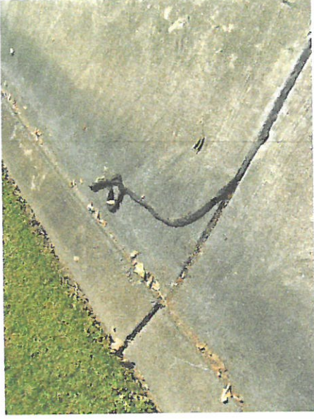
Dislodged joint sealant
