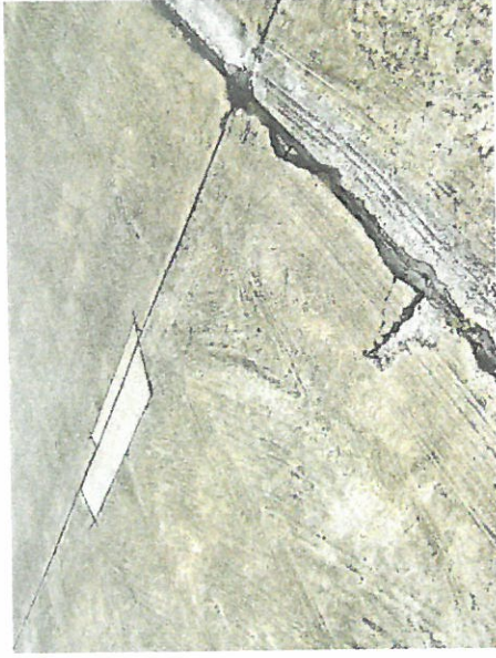
Previous patch and concrete spall at joint
