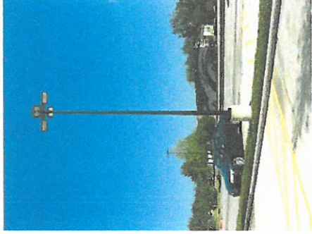
Light pole and fixture
